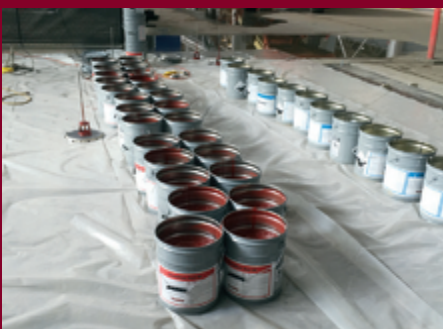
Chockfast Red HF Ready for Motor Mixer
